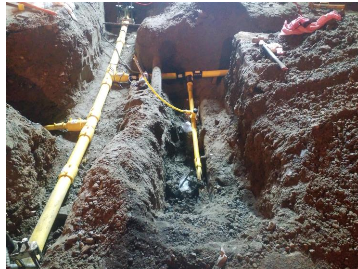
Figure 1: Major Leak on Waterloo Road
