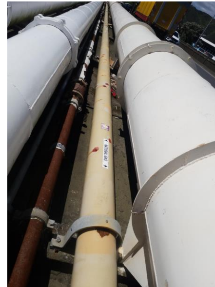
Figure 4: Corrosion on Waione Street Bridge Pipeline
