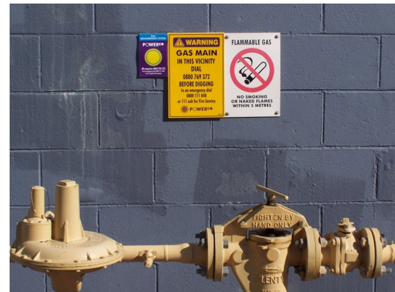
Figure 6.2: Example of Safety Signage.
