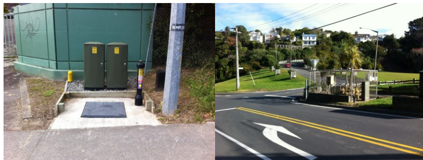
Figure 8.1: View of a Cocon Unit and an Above Ground Station.
