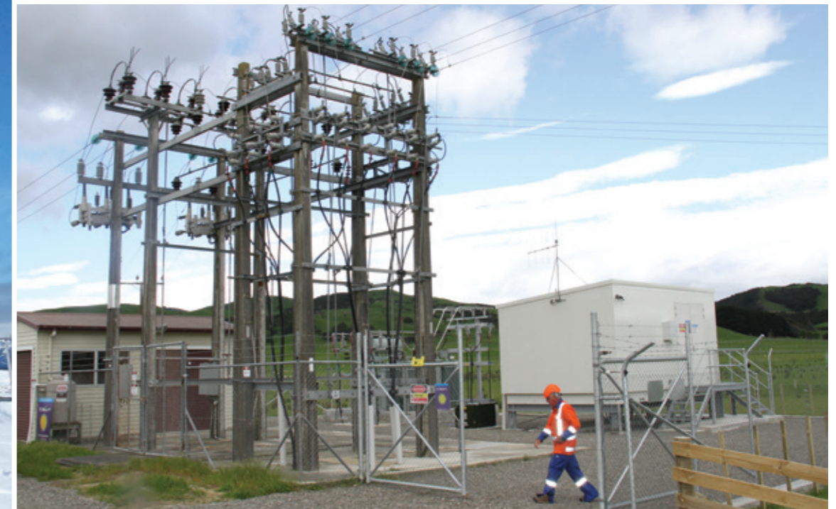
Below: To improve reliability of supply for remote Pongaroa customers, a $1 million project was undertaken to install new 11kV switchgear and replace the Pongaroa substation transformer.
