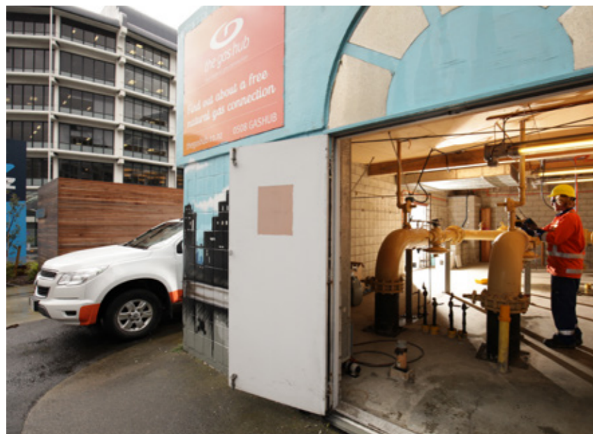
Below: To ensure we continue to deliver a safe and reliable gas supply to our customers, in the past year we began stage two of a project to significantly increase gas pressure in Wellington's CBD.
